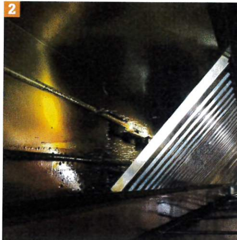
(2) Grease buildup covering a wet-chemical suppression system fusible link.
