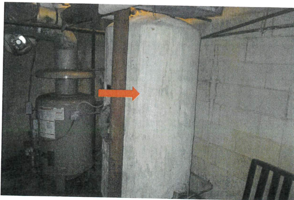
Figure 18: Looking at more TSI asbestos covering this water tank located in the basement of the vacant restaurant portion of the hotel.
