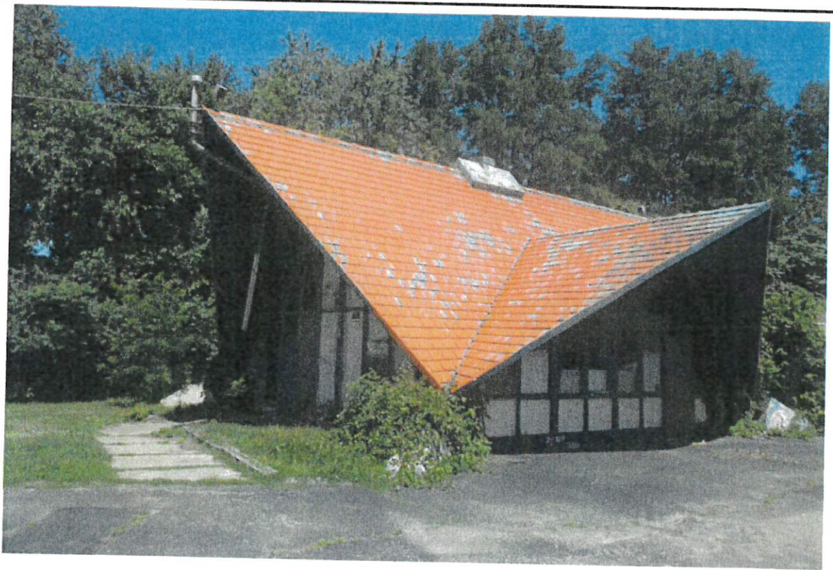
Figure 19: View of the front of the vacant former Howard Johnson's Motor Lodge building located on-site.
