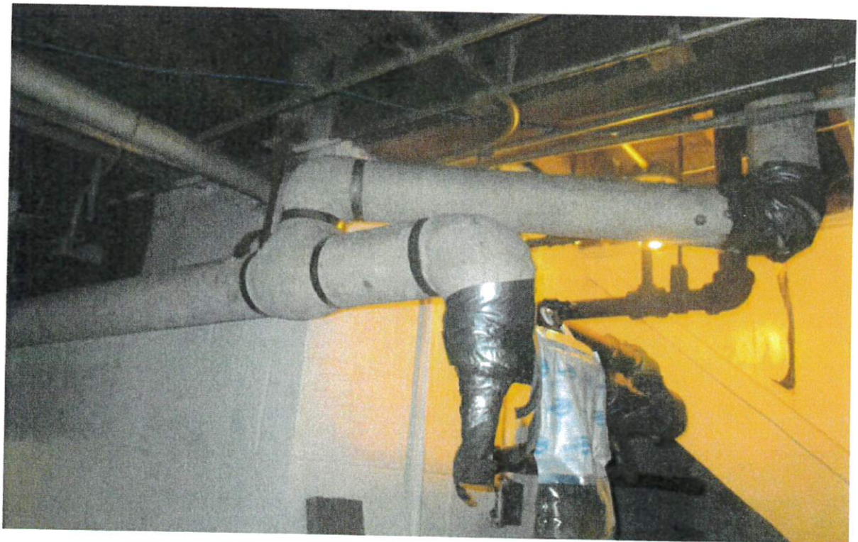
Figure 16: The physical site inspection revealed thermal system insulation (TSI) asbestos (above) located in the basement of the vacant restaurant portion of the hotel.
