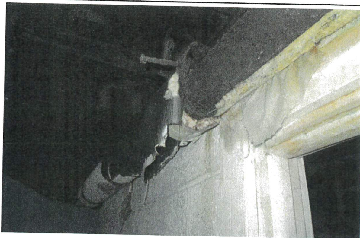
Figure 17: Some portions of the TSI asbestos (above) appear to be exposed, friable, and significantly damaged.
