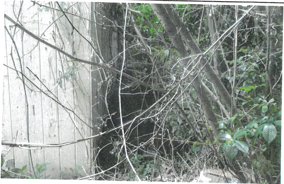
Figure 31: The physical site inspection was also hindered by dense vegetation (above) located along the rear walls of the former Howard Johnson's Travel Lodge building and the former Fischer World Travel building.
