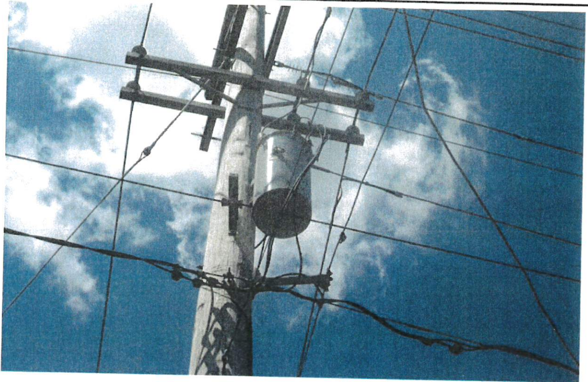
Figure 33: Looking at one of two pole-mounted electric transformers located on-site. No obvious visual evidence to suggest leakage was observed in the vicinity of the two electric transformers.
