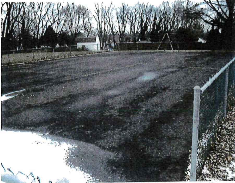
Existing Deteriorated Court
